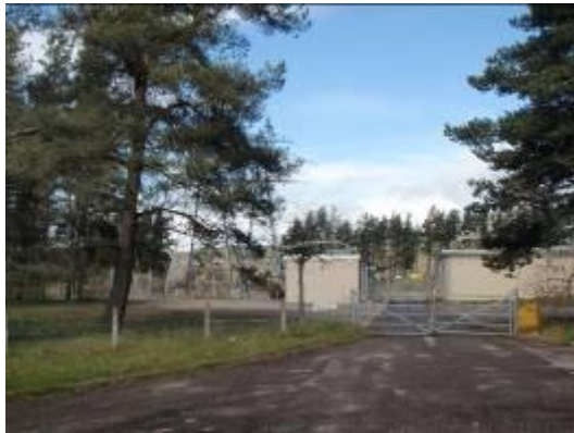
Fig 4: Boat of Garten substation
