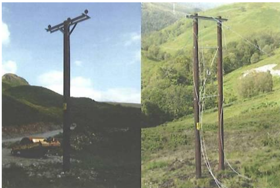
Fig. 3: Examples of single wooden pole and 'H' pole
